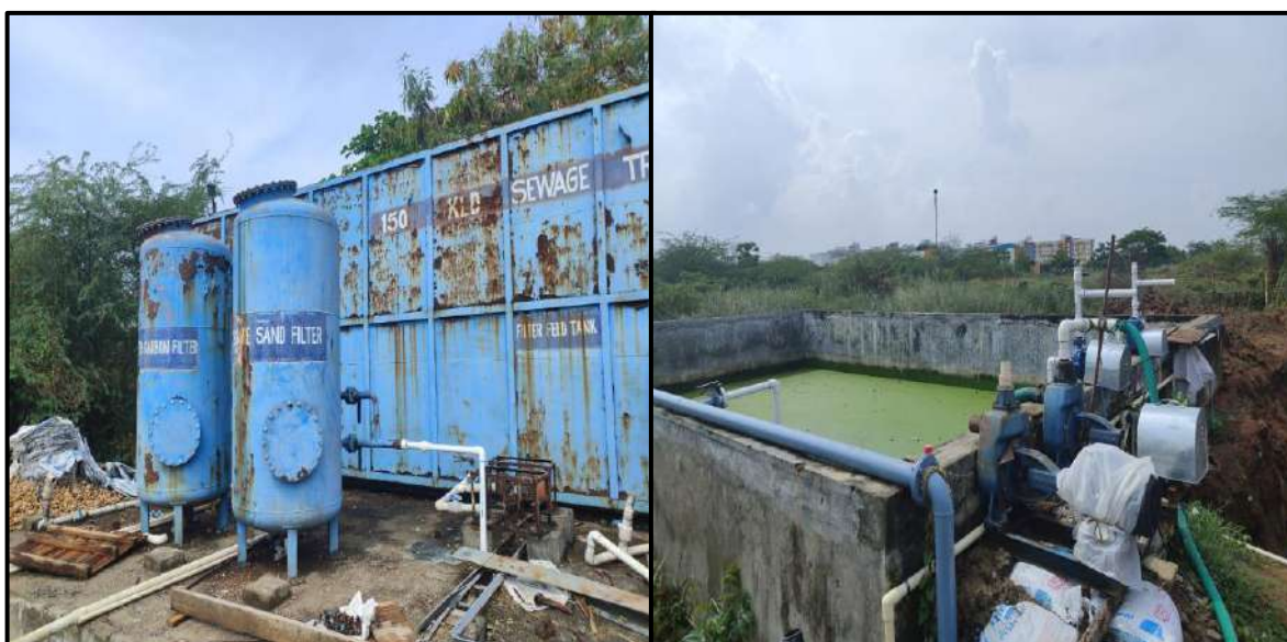
Sewage Treatment Units in Central University of Tamil Nadu, Thiruvavur, Tamil Nadu
